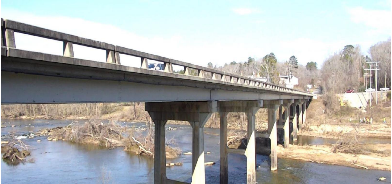
Figure C.3. A steel continuous multi-beam bridge with a reinforced concrete deck that was used as a case study to apply the developed tool.
